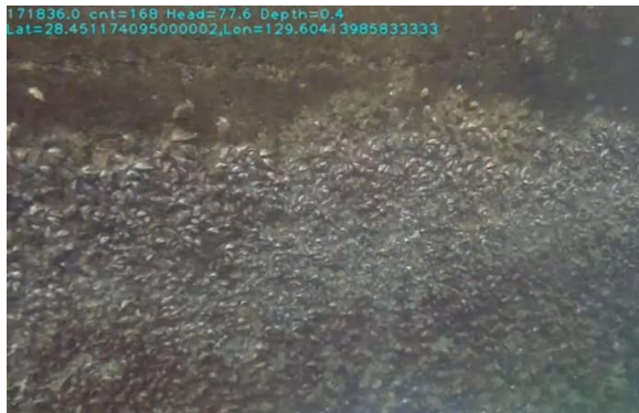
Fig.10 Concrete image captured by the AUV
