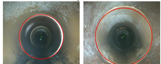
Fig.3. Pipe-joints and Hough transform results
